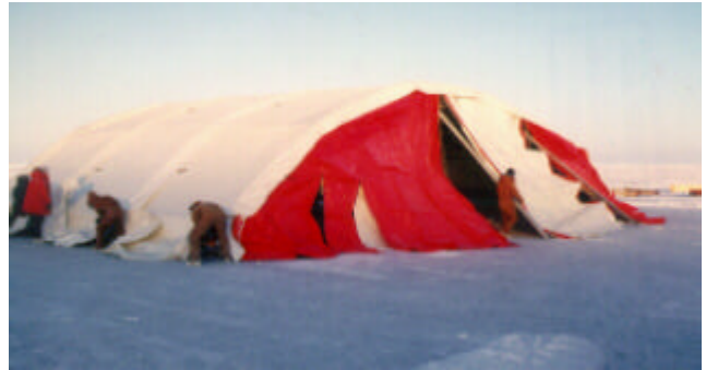
Figure 6. Wide Span tent going up. Note the four people on the left cranking up the tent with boat winches.
